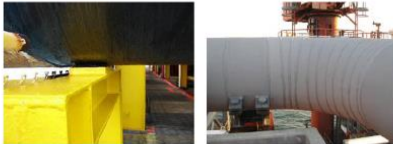
Figure 10 Example of good versus poor implementation of corrosion controls observed during a visual audit conducted by the HSE. (Health & Safety Executive 2010, 23)
