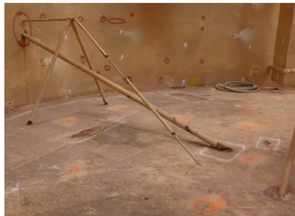
Figure 4 – A failed oxygen sparge has made contact with the floor and through movement caused by the agitation of the slurry is mechanically removing the coating on the
