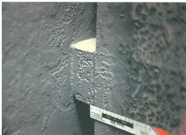
Figure 7 – View shows minor pitting in an area of increased velocity close to a baffle support. Image was taken after abrasive cleaning
