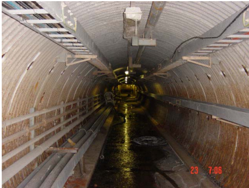
Fig II: General view of Escape Tunnel prior to refurbishment. Note the corrosion degradation at the lower third of the tunnel.
