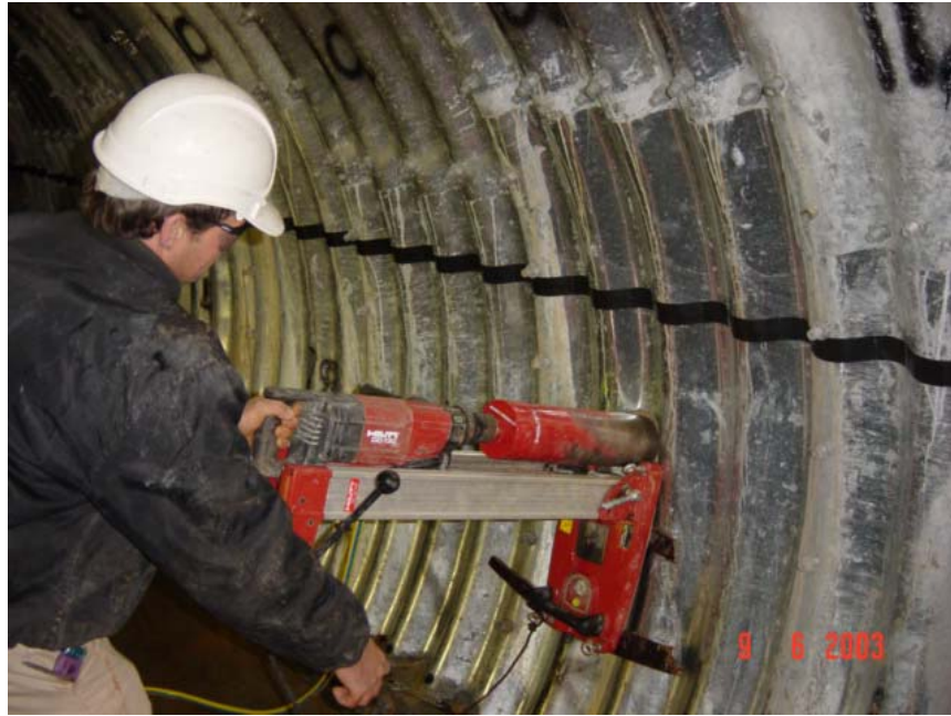
Fig XII: Photograph showing coring activity through tunnel walls with diamond tipped core to facilitate anode placement.
