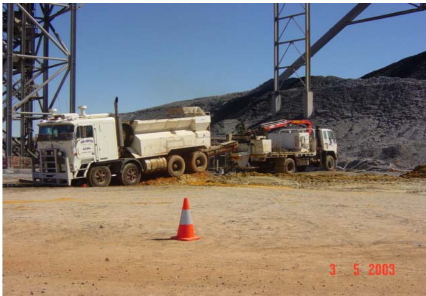
Fig IX: View of grouting truck arrangement. Concrete was batched on-site due to remoteness and pumped directly into spray unit hopper.
