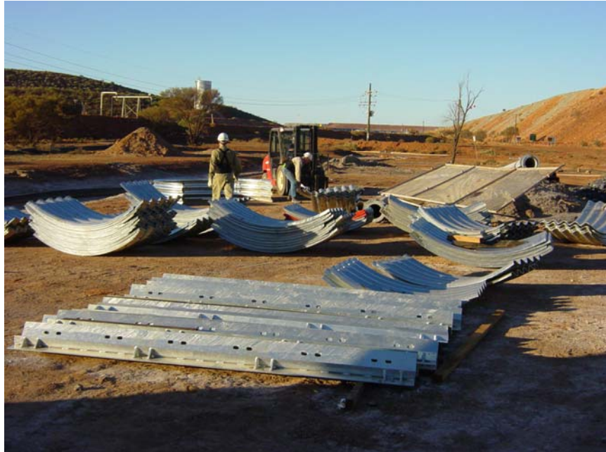
Fig VII: Photograph showing new tunnel sections and fabricated angle bases as unloaded on-site.
