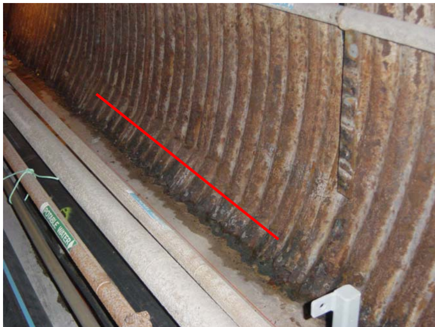
Fig III: Close up view of corrosion degradation typical in the Escape Tunnels. Note also kink in the tunnel wall above red indicator line.
