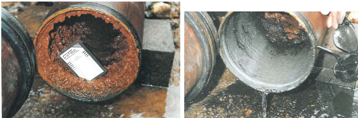
Fig.1 A/B – Condition of the HDG pipe on opening and after removal of tubercles
