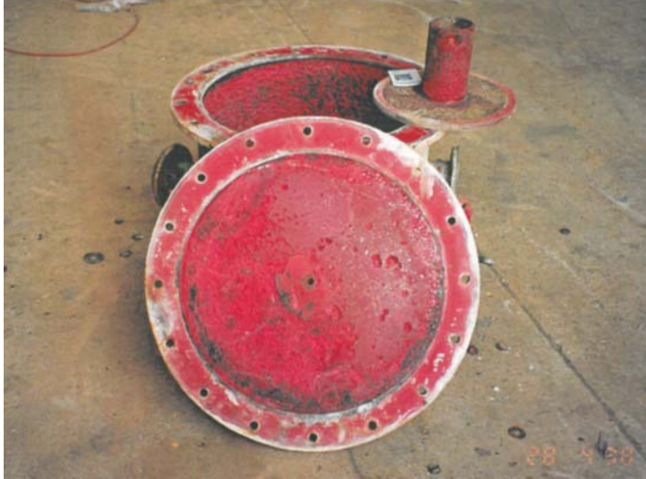
Fig 3A – General view of rubber lined Cyclone cover, badly affected by deterioration of the natural rubber lining used for internal protection.
