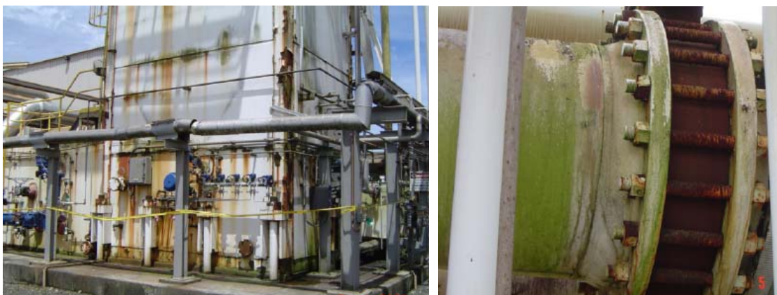
Fig 4 A/B – Algal growth over the high build epoxy on an Oxygen plant cooling tower, including the piping.
