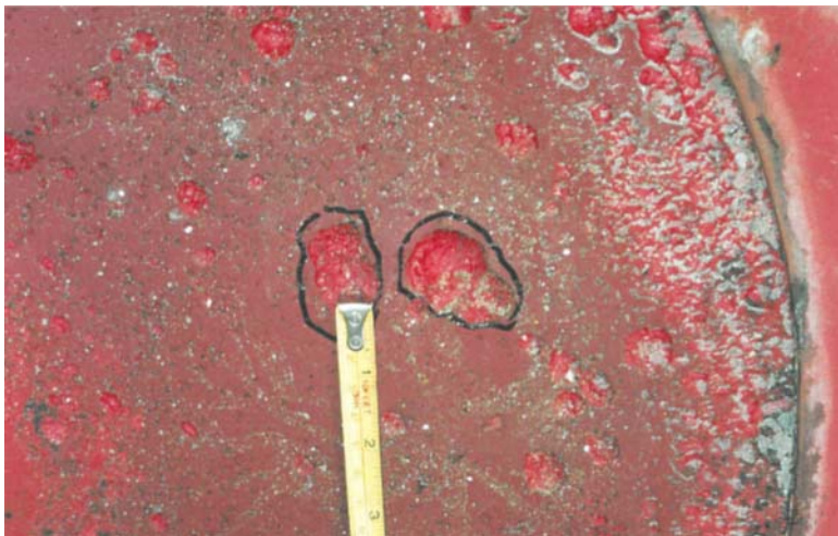
Fig 3B – Close up of the rubber lined Cyclone cover, showing the “pitting” as the rubber deteriorated, prior to the exposure of the underlying steel and the MIC associated with the substrate steel.
